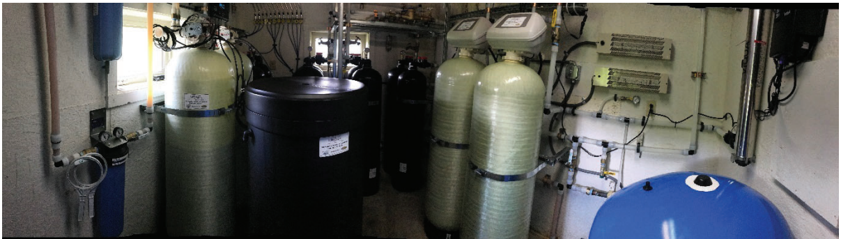
Exhibit 2-3: Installed point of entry treatment system
